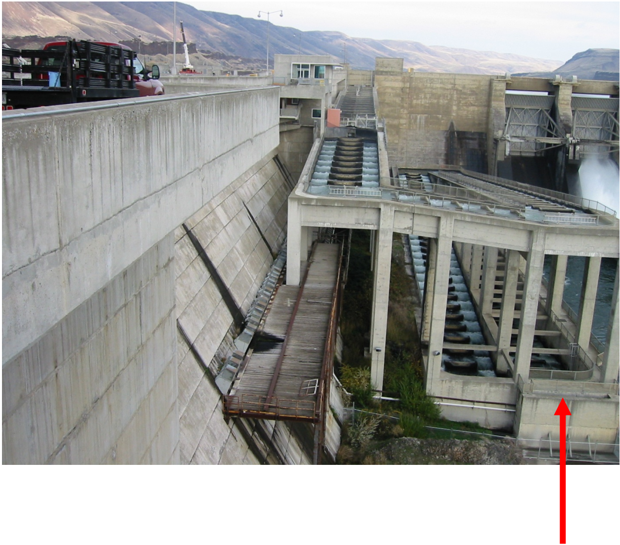
Photo 2. End view of North Fish Ladder – the AWS vent-well is shown in the lower right corner, as a projection from the end turn of the fish ladder channel, per the arrow. Three struts are at the base of the AWS vent-well wall.
