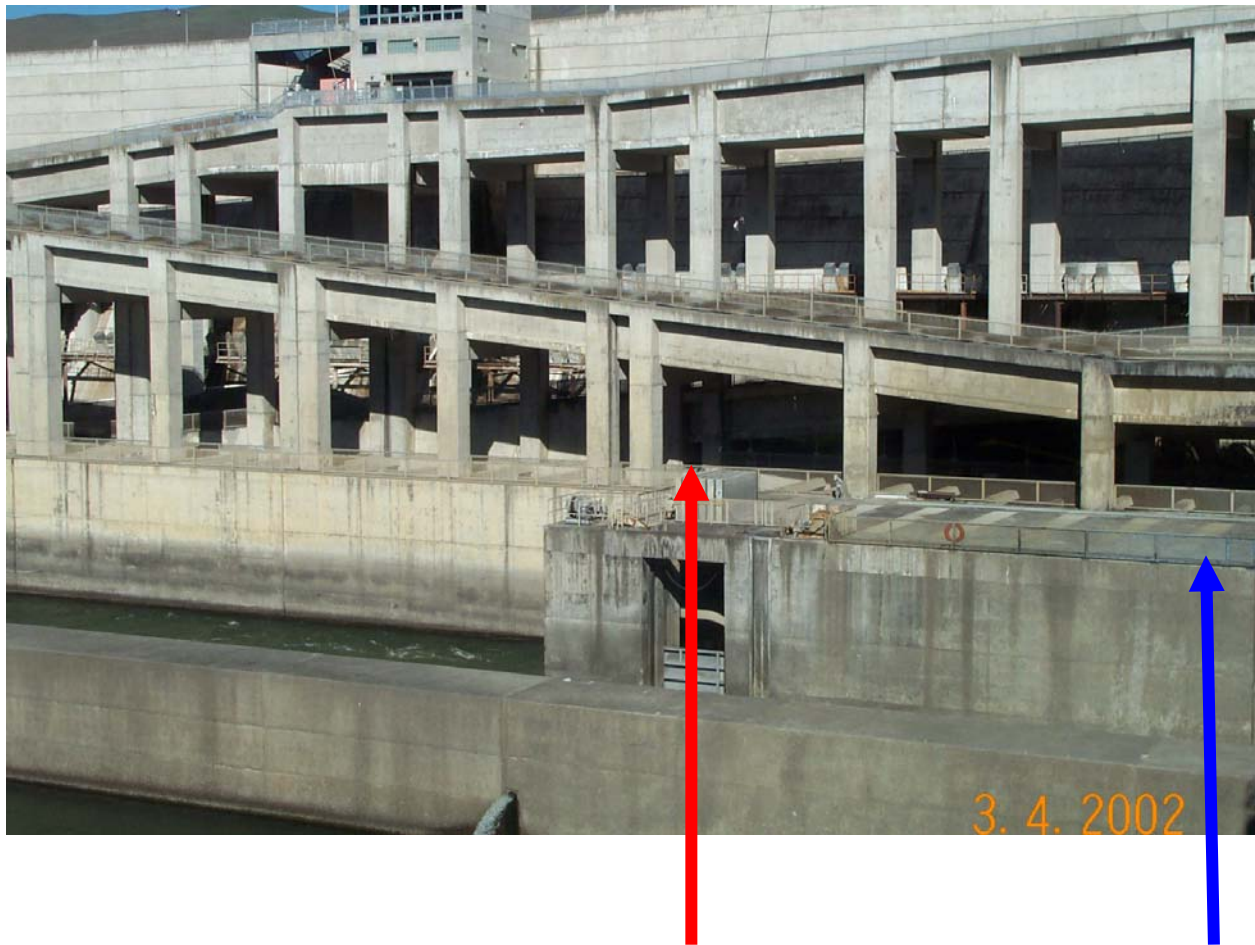
Photo 4. Elevation view of N Fish Ladder – the fish channel transect is located just right of the closely spaced dual concrete columns in line-sight with the entrance end of the fish ladder. The monolith joint runs between the two closely-spaced columns. The fish channel transect is nine feet to the right of the monolith joint, lying just to the right of right column as noted by the red arrow. The blue arrow pointing to the Elev. 185 deck is where e-tape water-surface level indicators are used to determine the water surface, just within the fish ladder entrance.
